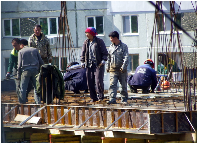
North Koreans working on a construction site in Vladivostok, 2016. Photo by Leonid Kozlov.
